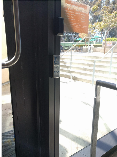
Figure 3. Handicapp door opener that opens into a stair-protected foyer.
